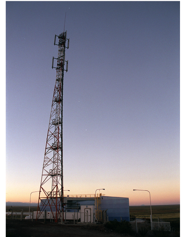
Fig. 12. One of the five communications towers: the one shown is deployed at the Los Leones site; see Fig. 11.
